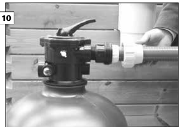
10 The pump and filter are interlinked by a semi-flexible tube.
