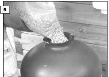
5 Fill the filter first with gravel (3-5mm) and then with sand (0.4-0.8mm). The sand has an unlimited lifetime and only need to be topped up in case sand is lost. Mark the level of sand/gravel to be able to re-fill the filter to the correct level at a later time.
